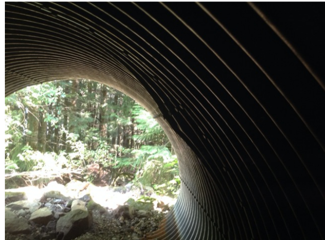
inside minor damage
